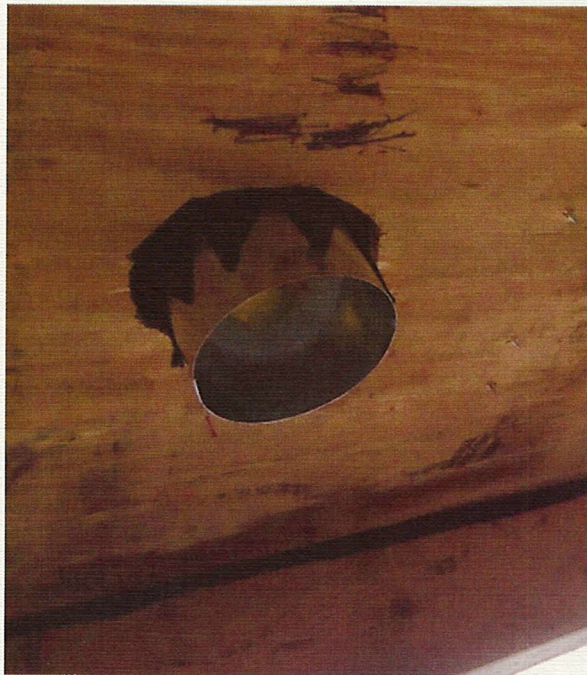
BELOW DECKING WITH 4" DIAMETER EXTENDED PIPING
